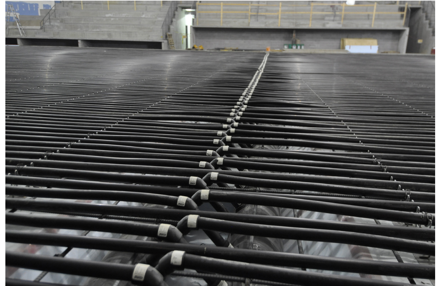
Ice Slab Refrigeration Lines
