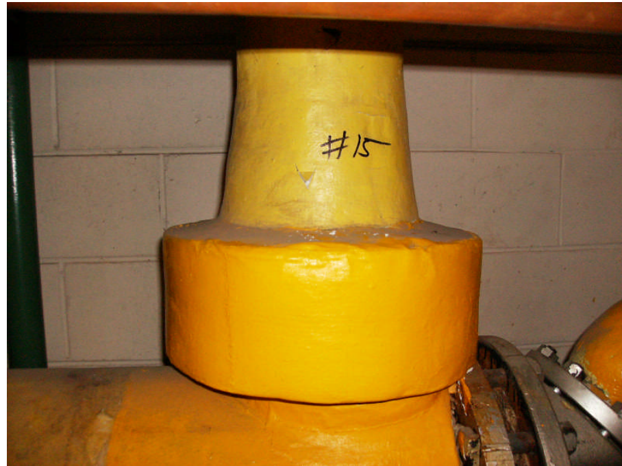
FIGURE 12: Grey Asbestos Containing Pipe Fitting Insulation
