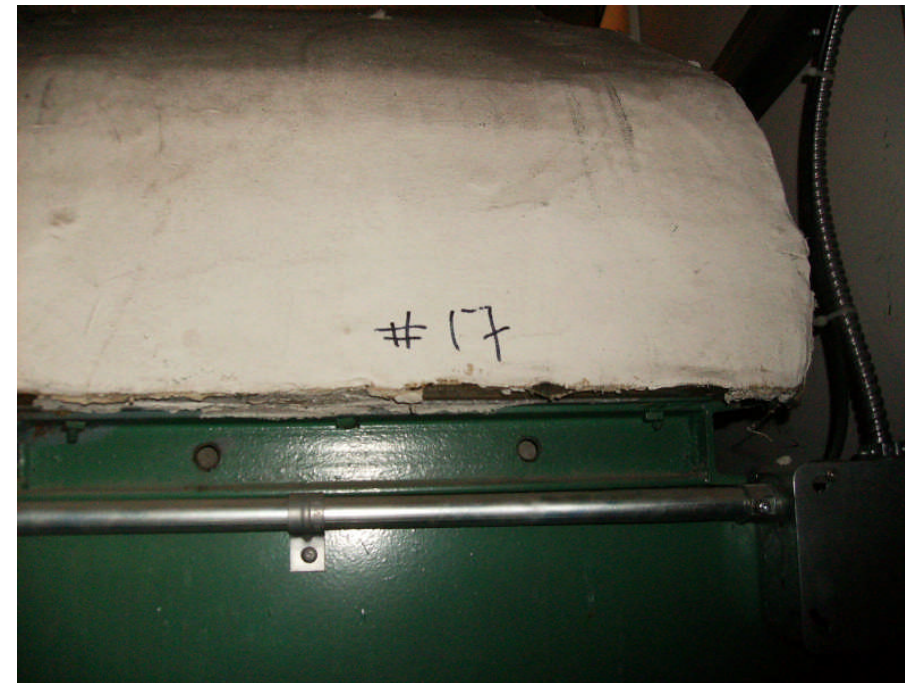
FIGURE 14: Grey Asbestos Containing Parging Mud on Duct
