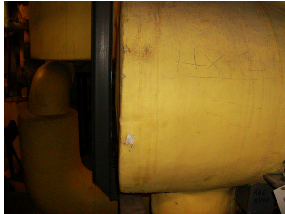
FIGURE 10: Grey Asbestos Containing Parging Mud On Tank
