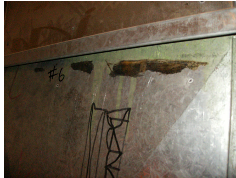
FIGURE 3: Black Asbestos Containing Mastic on Duct
