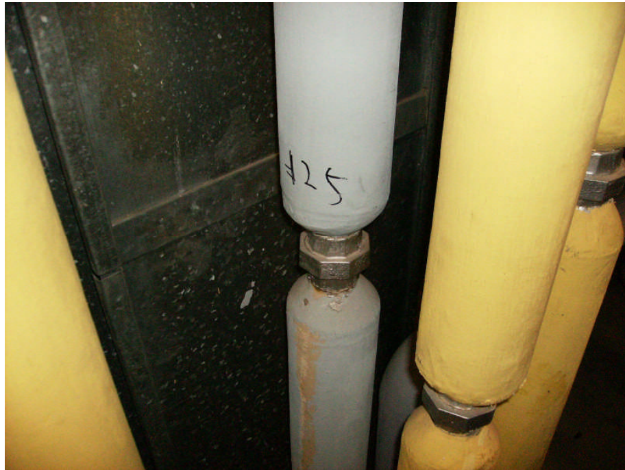
FIGURE 23: Grey Asbestos Containing Valve Fitting Insulation
