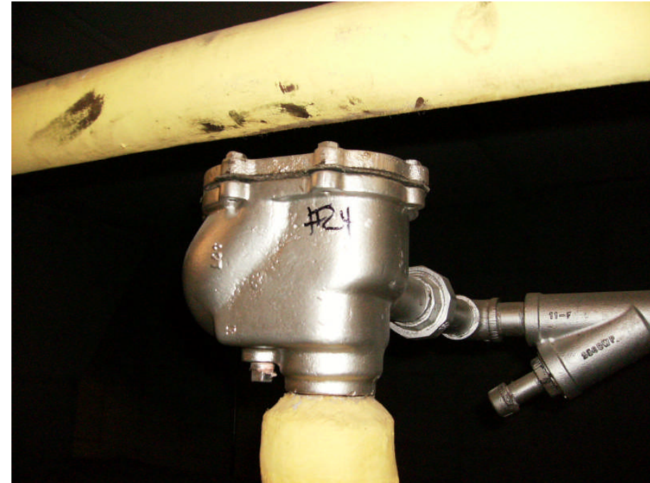
FIGURE 22: Black Asbestos Containing Gasket
