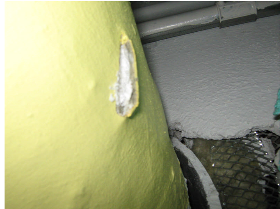
FIGURE 6: Grey Asbestos Containing Pipe Run Insulation
