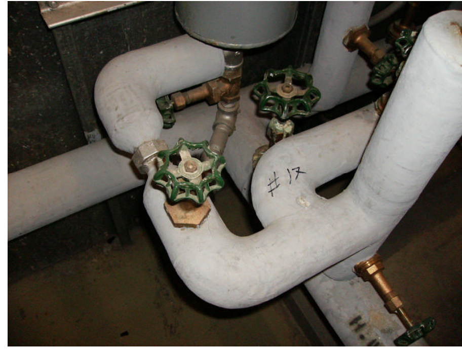
FIGURE 17: Grey Asbestos Containing Pipe Fitting Insulation
