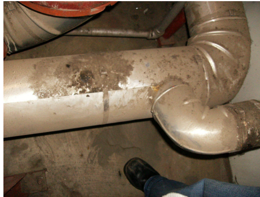
FIGURE 5: Brown Asbestos Containing Parging Under Metal Cladding
