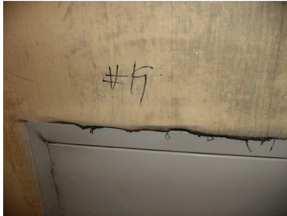
FIGURE 19: Grey Asbestos Containing Parging Mud on Duct
