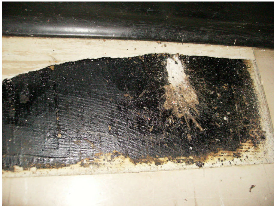
FIGURE 24: Grey Asbestos Containing Floor Leveling Compound (Cement) with Black Mastic
