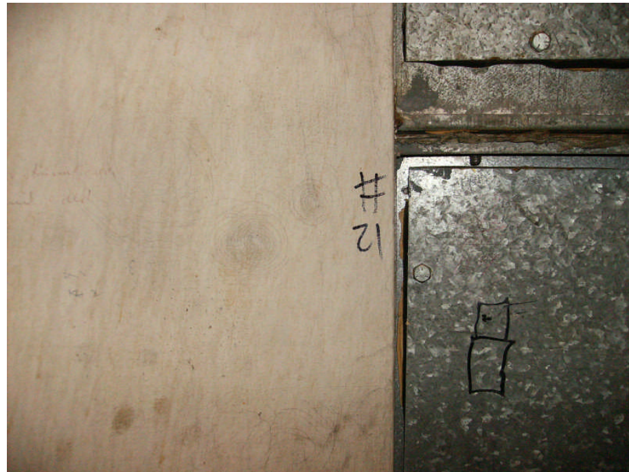
FIGURE 20: Grey Asbestos Containing Parging Mud on Duct
