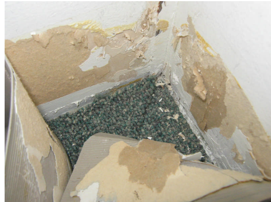
FIGURE 6: Beige Asbestos Containing Drywall Joint Compound
