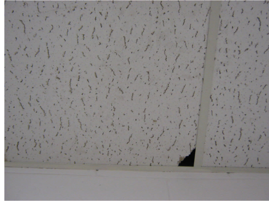
FIGURE 5: Grey Asbestos Containing Ceiling Tile (2x4)
