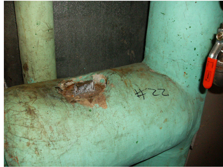
FIGURE 21: Grey Asbestos Containing Pipe Fitting Insulation
