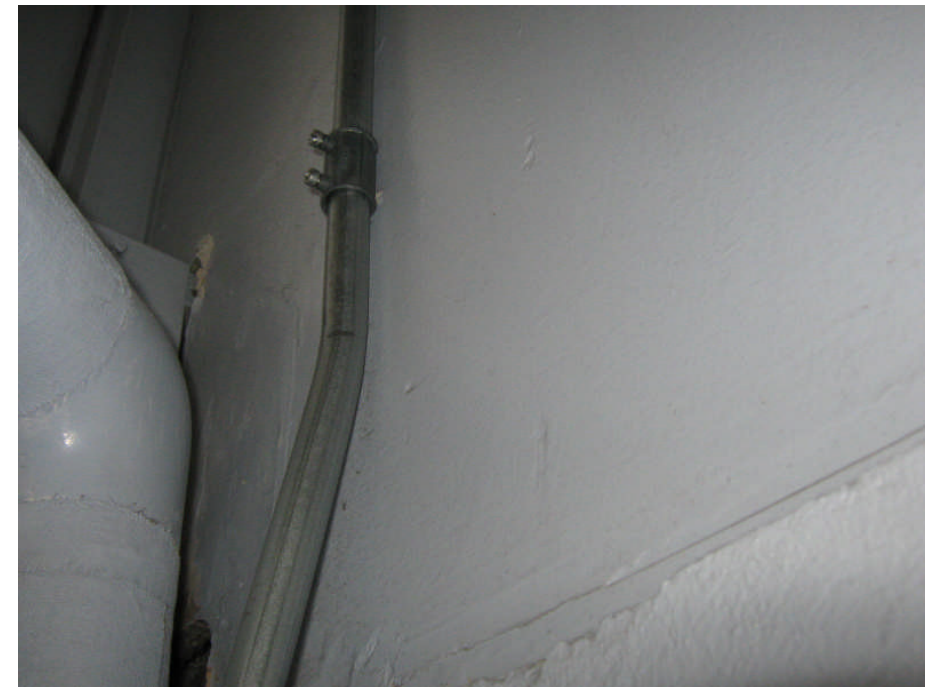
FIGURE 2: White Asbestos Containing Drywall Joint Compound
