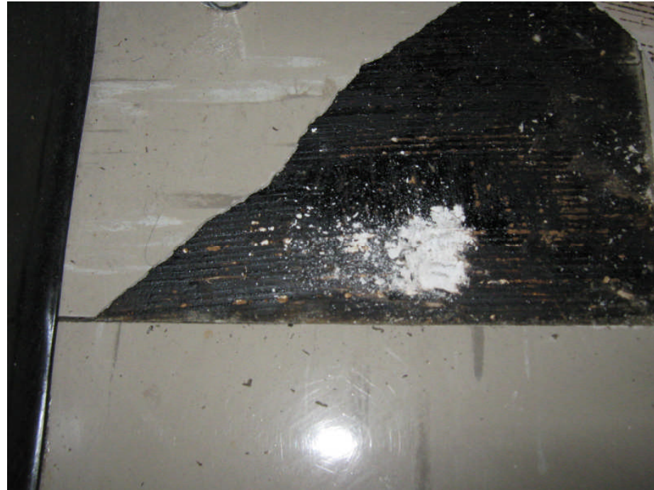
FIGURE 4: White Asbestos Containing Floor Levelling Compound (cement-like)
