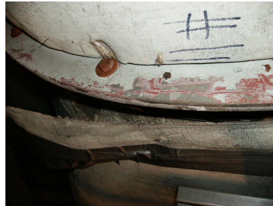
FIGURE 14: Grey Asbestos Containing Parging Mud on Duct
