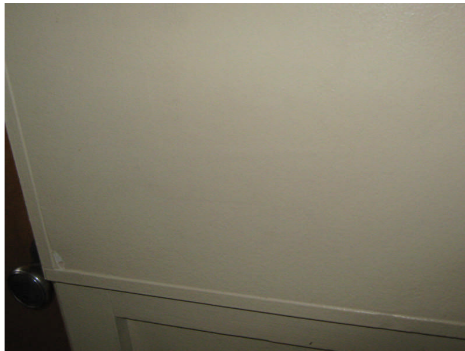
FIGURE 8: White Asbestos Containing Drywall Joint Compound
