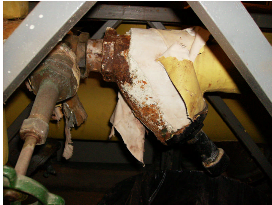
FIGURE 11: Grey Asbestos -Containing Valve Fitting Insulation
