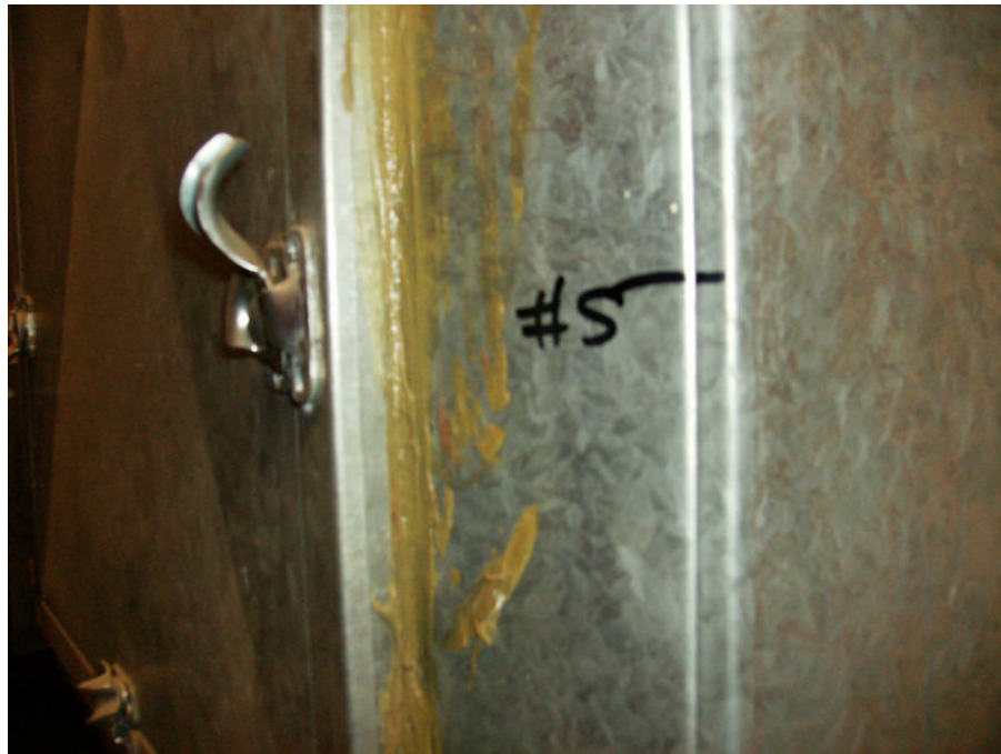
FIGURE 2: Amber Asbestos Containing Mastic on Duct
