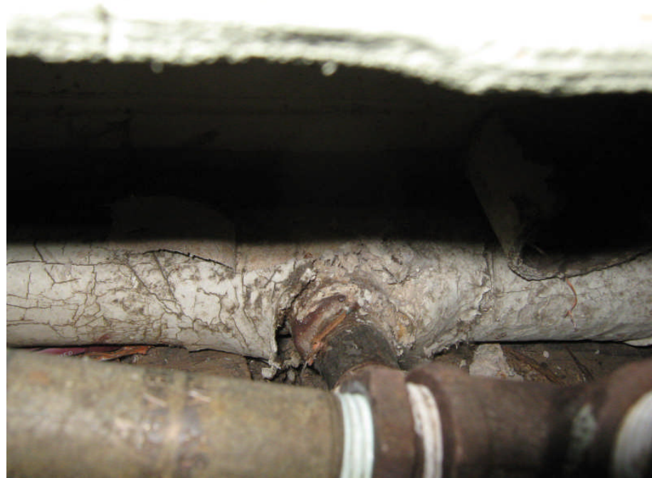
FIGURE 7: Grey Asbestos Containing Pipe Fitting Insulation
