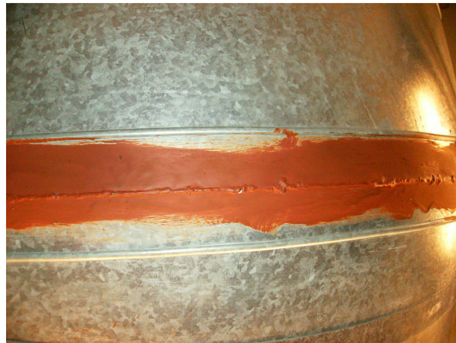
FIGURE 6: Red asbestos-containing mastic on duct.
