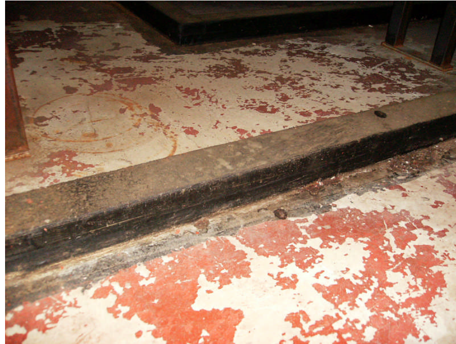
FIGURE 15: Black Asbestos Containing Floor Mastic
