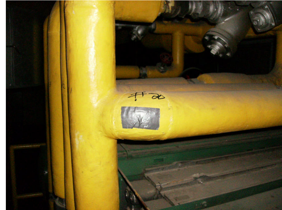
FIGURE 17: Grey Asbestos Containing Pipe Fitting Insulation
