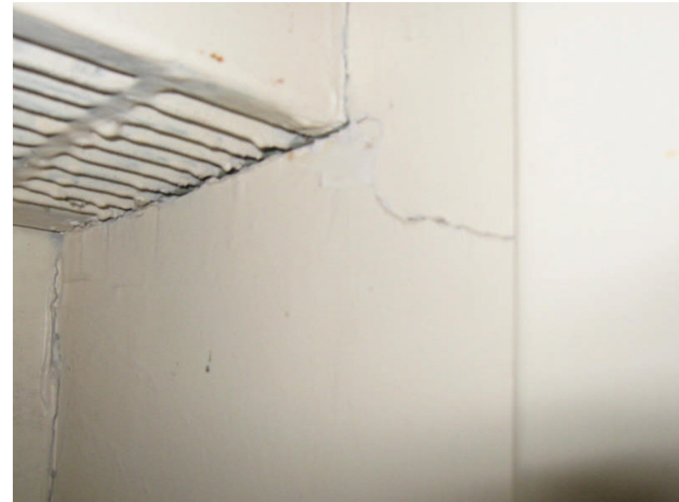
FIGURE 9: White Asbestos Containing Drywall Joint Compound
