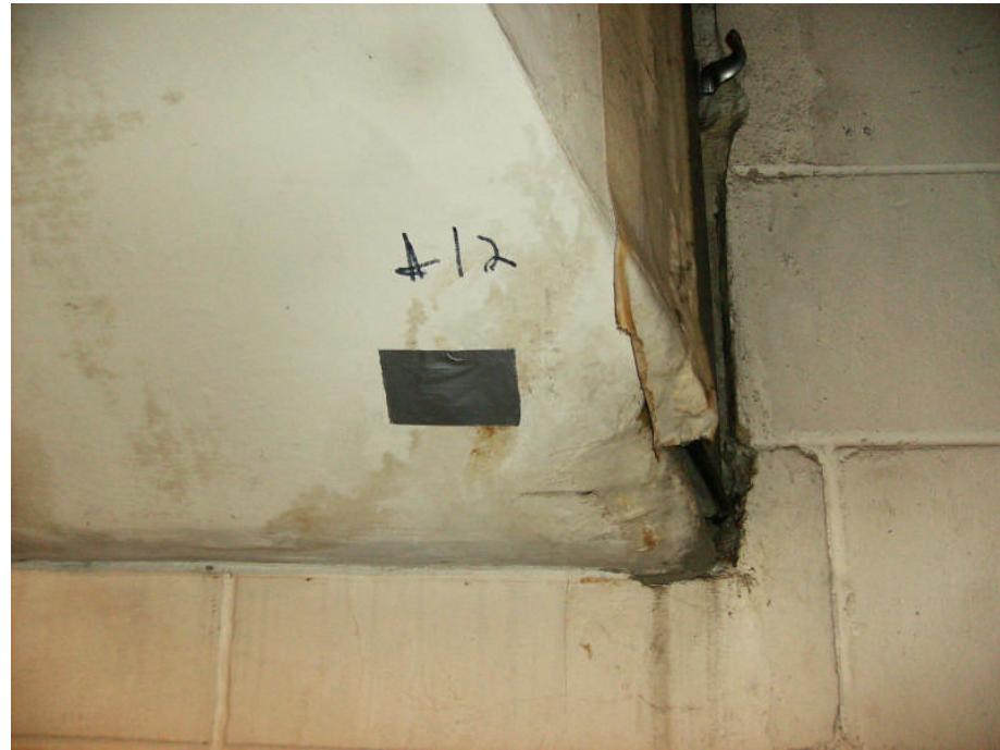
FIGURE 11: Grey Asbestos Containing Parging Mud on Duct
