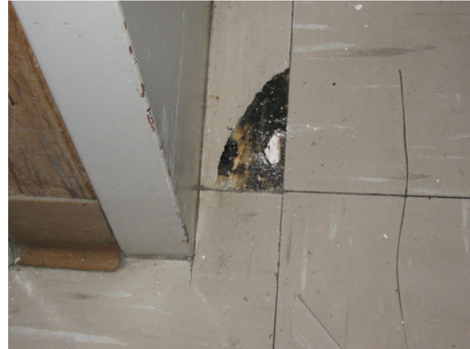
FIGURE 5: White Asbestos Containing Floor Levelling Compound (cement-like)
