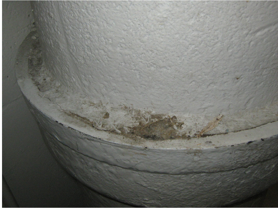
FIGURE 1: Brown Asbestos Containing Cast Iron Joint Packing
