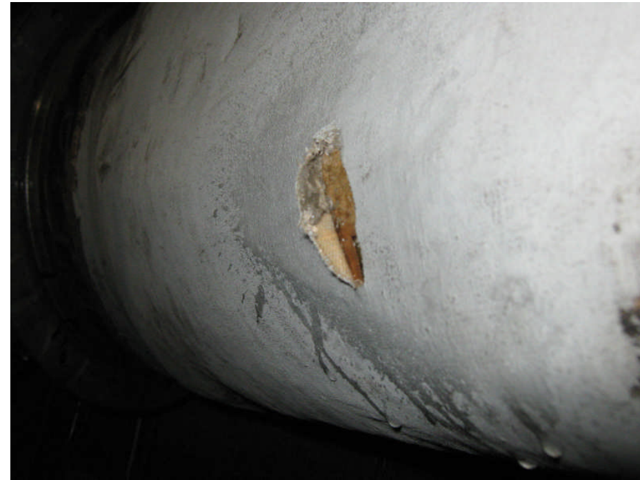
FIGURE 1: Grey Asbestos Containing Parging Mud on Duct
