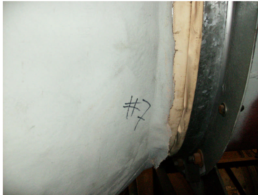
FIGURE 12: Grey Asbestos Containing Parging Mud on Duct
