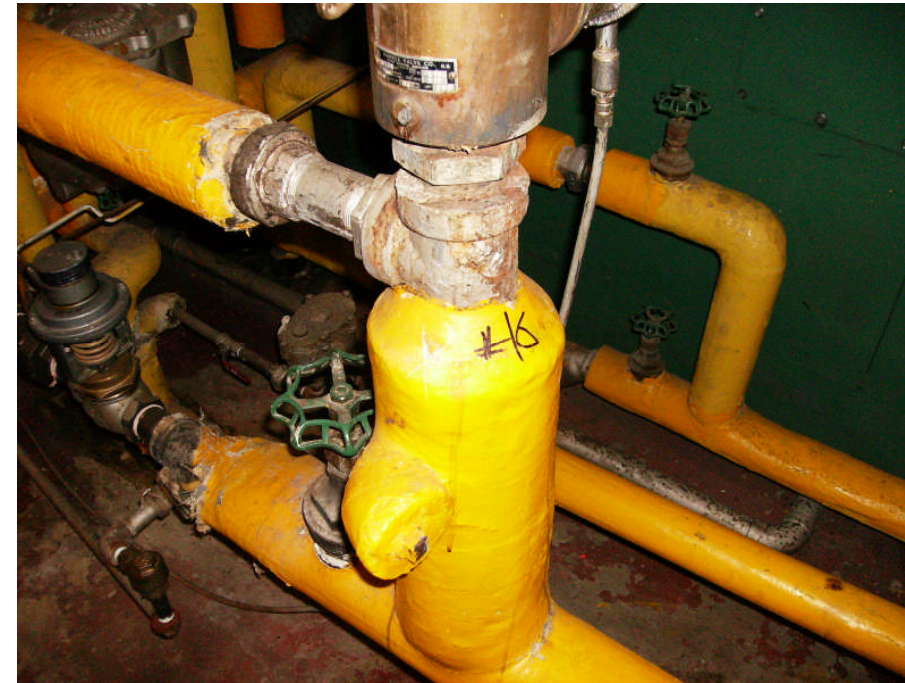
FIGURE 13: Grey Asbestos Containing Pipe Valve Insulation
