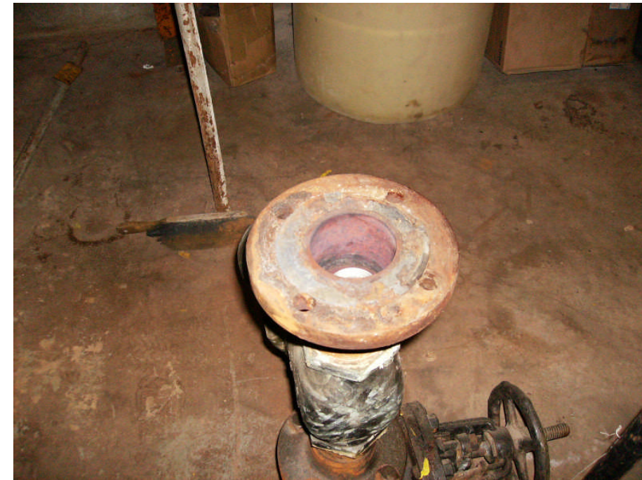
FIGURE 18: Black Asbestos Containing Gasket
