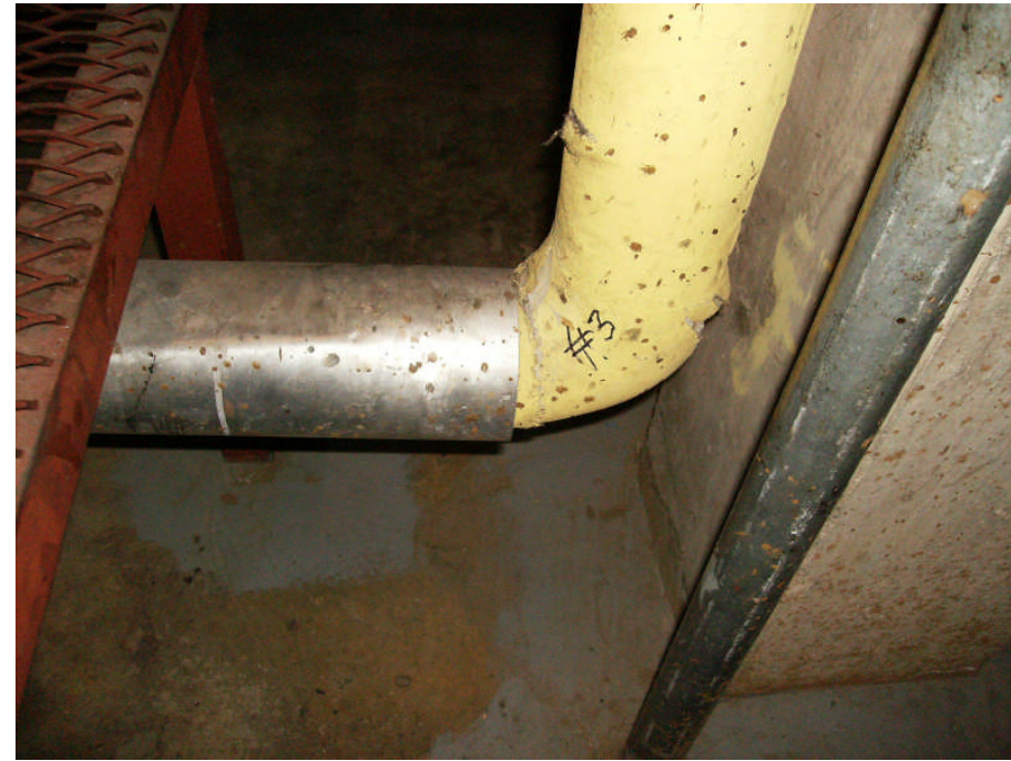
FIGURE 9: Grey Asbestos Containing Pipe Fitting Mud on 4" Yellow LPC Line
