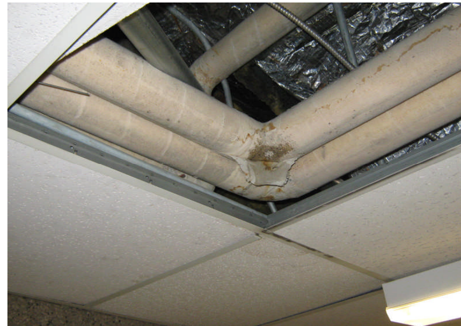
FIGURE 2: Grey Asbestos Containing Pipe Fitting Insulation
