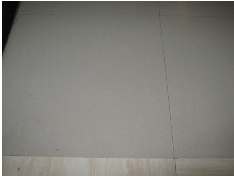
FIGURE 7: White Asbestos Containing Floor Levelling Compound (cement-like)
