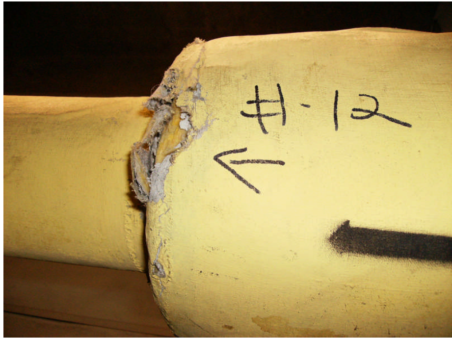
FIGURE 15: Grey Asbestos Containing Valve Fitting Insulation
