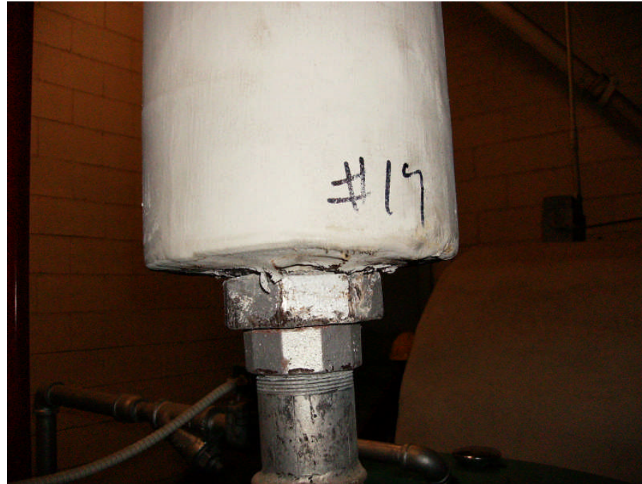
FIGURE 16: Grey Asbestos Containing Exhaust Parging
