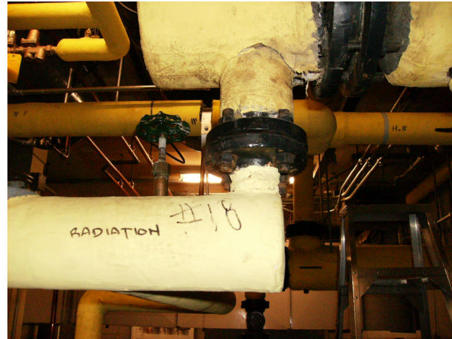
FIGURE 18: Grey Asbestos Containing Valve Fitting Insulation
