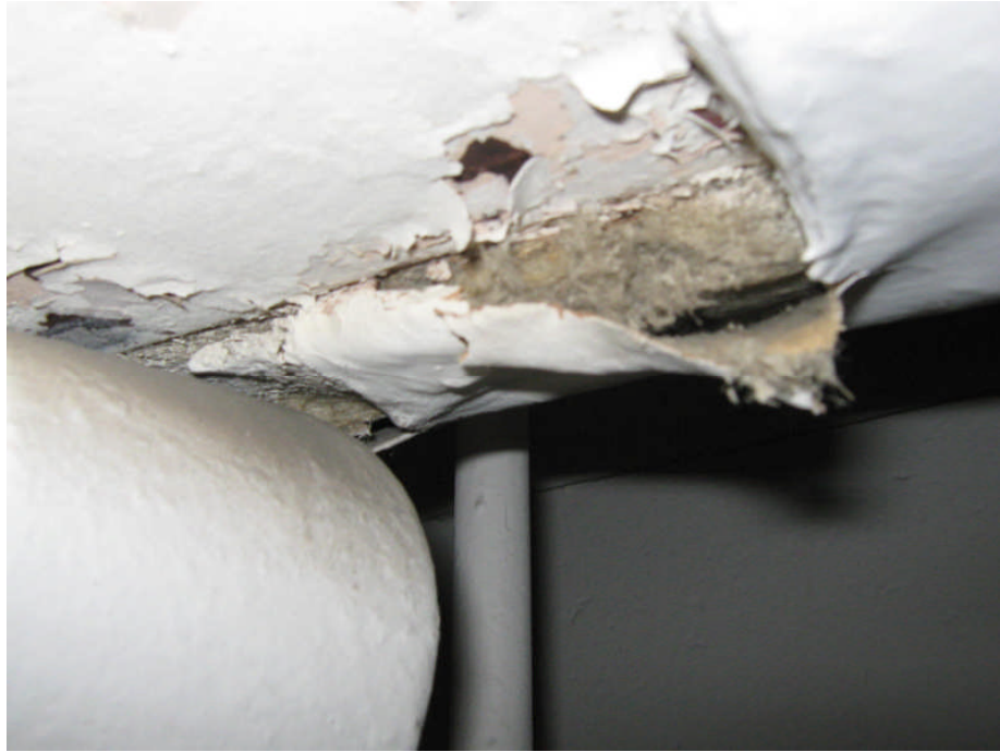
FIGURE 3: Grey Asbestos Containing Pipe Run Insulation
