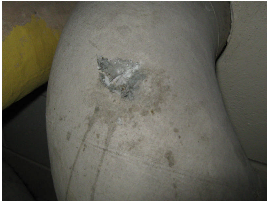
FIGURE 4: Grey Asbestos Containing Pipe Fitting Insulation
