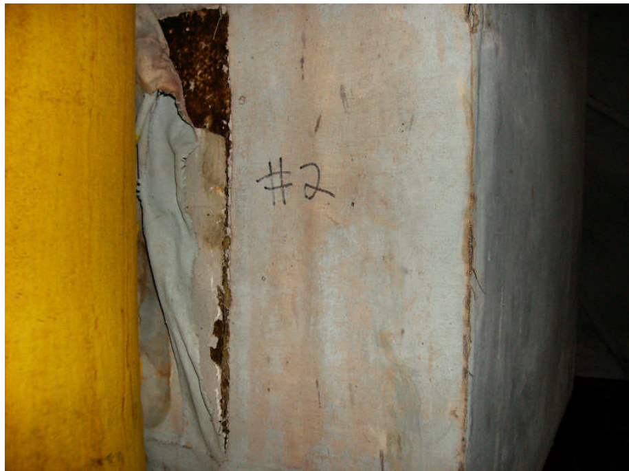
FIGURE 8: Grey Asbestos Containing Parging Mud on Duct
