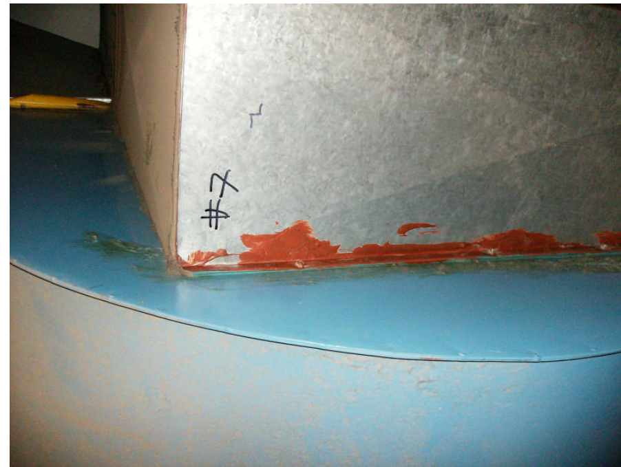
FIGURE 4: Red Asbestos Containing Mastic on Duct
