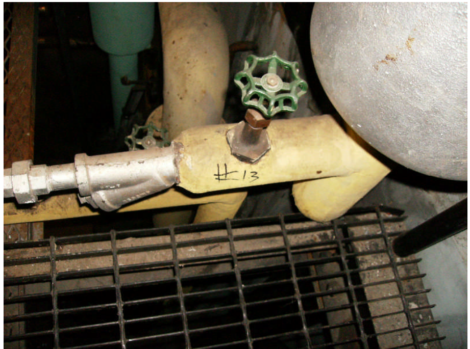
FIGURE 16: Grey Asbestos Containing Pipe Fitting Insulation
